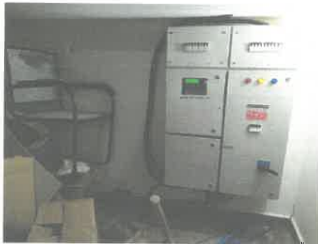
Electrical room should be provided with ventilation and free from all possible dumps.
