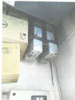
Batteries stacked for disposal (typical).
